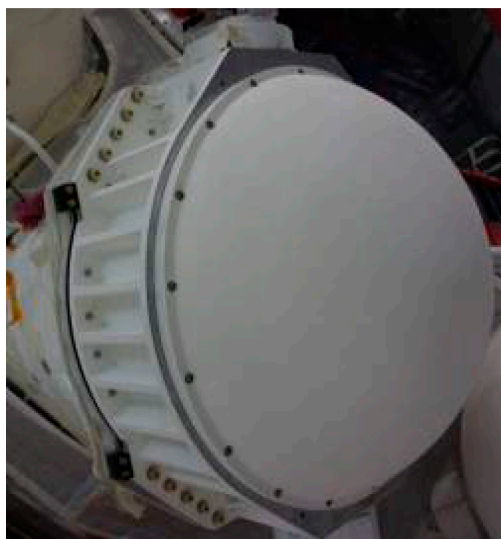
A Outside installation
